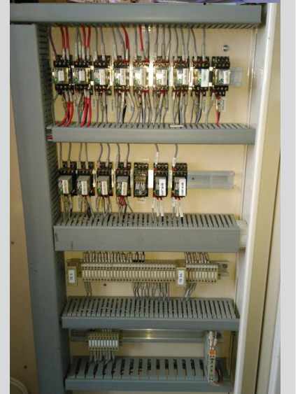
Figures 1, 2 & 3: Legacy DCS and control cabinet wiring that required detailed inspection during the site survey.
