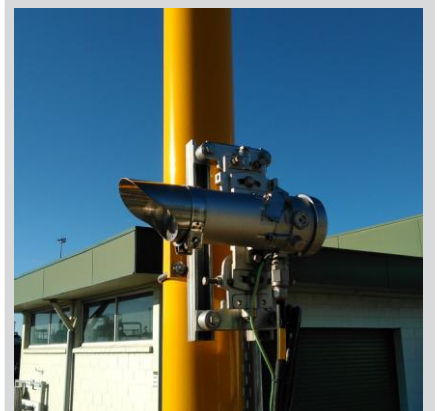
Representative fire and gas detection technologies considered during performance-based coverage evaluation.
