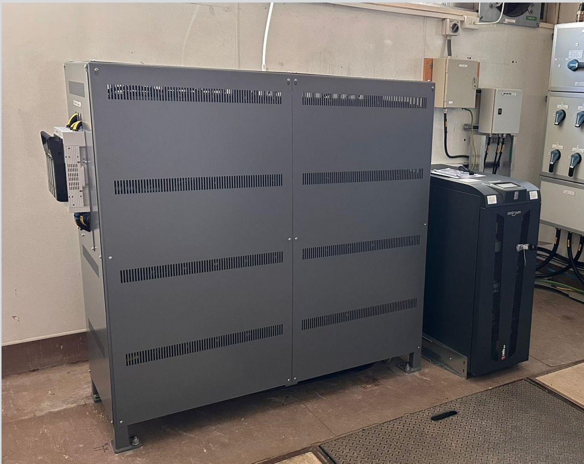
Figure 4: Upgraded 60 kVA UPS and Battery Bank
