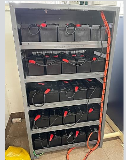
Figures 1 & 2: Legacy UPS and battery bank within the replacement scope.
